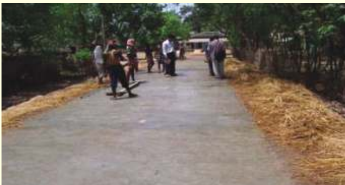
Fig 5. A finished surface of the concrete road after removal of paddy straw used for wet curing
